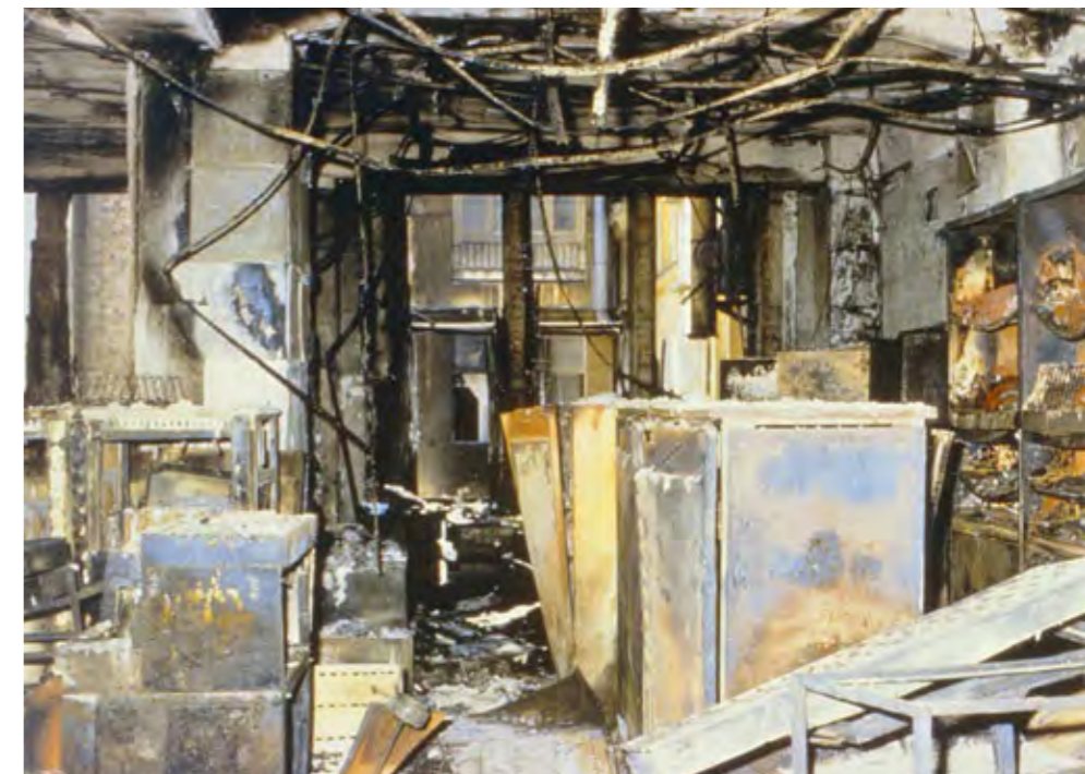
Images from a Central Bank building fire
